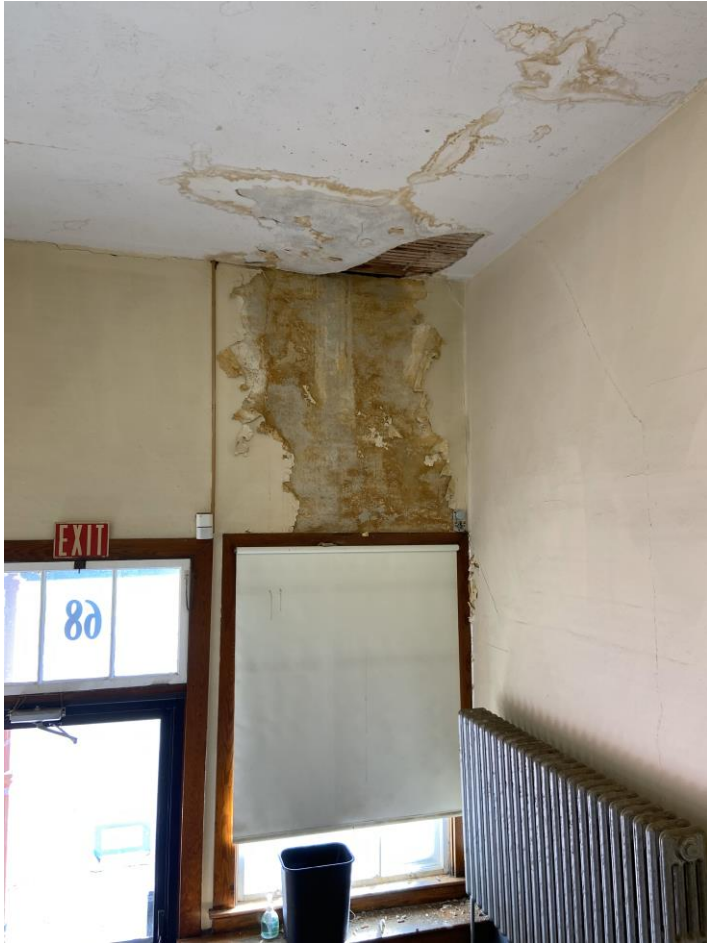
Extensive water damage, Annex Entryway
