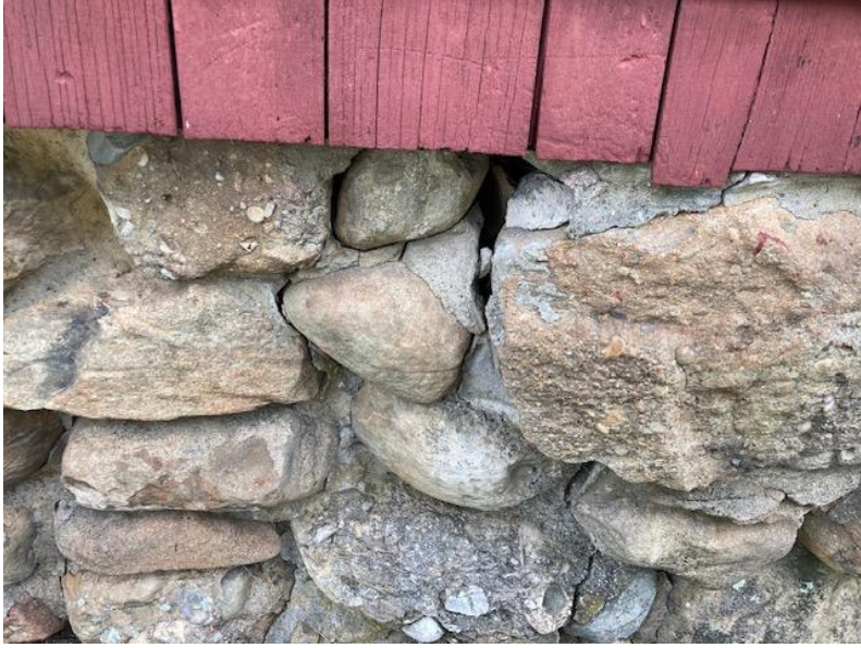
Deficiencies in Foundation, Town Hall Annex
