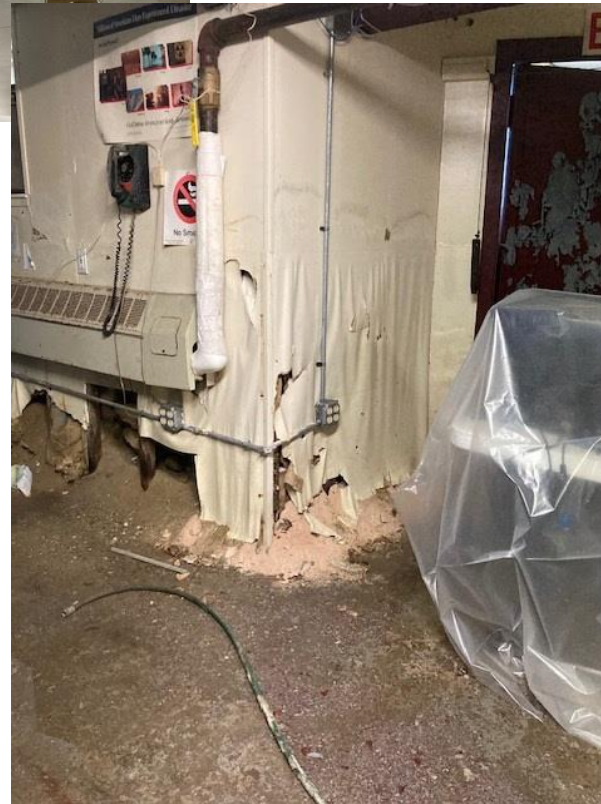
Water damage, basement
