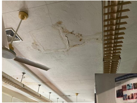
Water damage, Ceiling, Veterans Office
